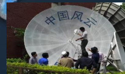
FY-2H DB Station Installation in Bangladesh
